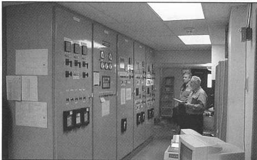
The power plant's paralleling switchgear allows for both power import and export. The switchgear was manufactured by Prime Automation and features several Basler generator monitoring components. Engine monitoring and control is via a Deutz total electronic management (TEM) system.
